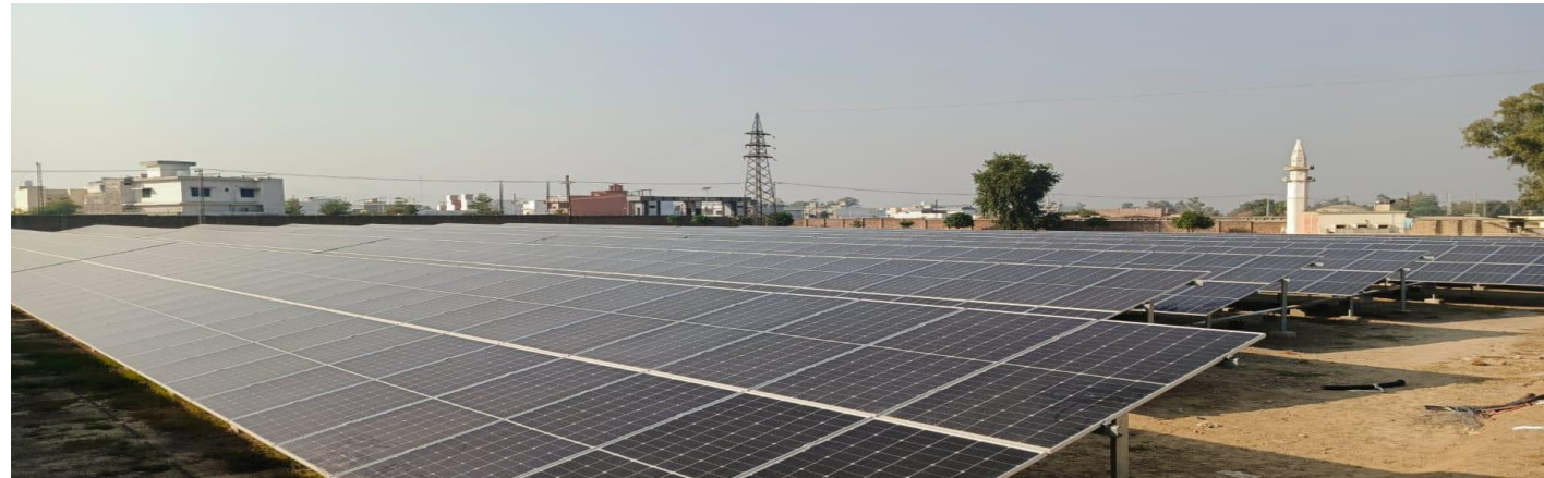
Another one-megawatt solar power plant under final stages of installation, financed through SBP Renewable Energy Scheme.
