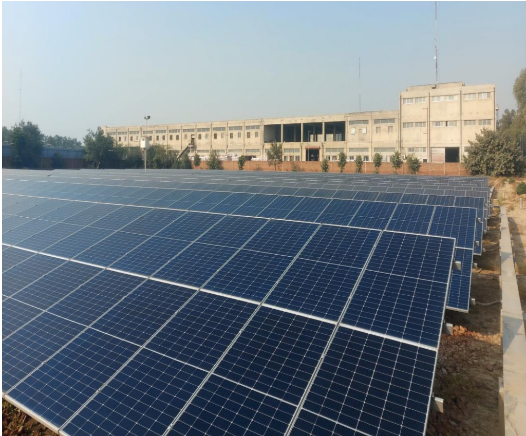
One-megawatt solar power plant fully operational.
